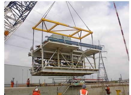
Typical gantry used on CTRL
