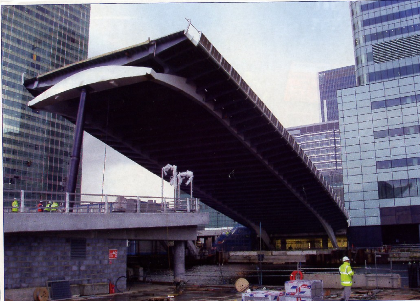
ON THE UP: The first full lift of the Great Wharf Road in London's Docklands took place recently. The 1,100t road bridge, designed by Gifford and Wilkinson Eyre, was lifted by a Hunger Hydraulik two-stage telescopic hydraulic ram. Bennett Associates, the design team's M&E consultant, claimed it is the UK's largest hydraulic ram. It extended to its full length of 18m to lift the bridge about its pivot bearings, providing access through the North Dock to and from West India Quay. The bridge opens to traffic next month.
